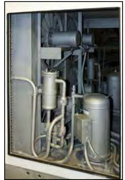
Close-up view of a Carboline-coated condenser section
